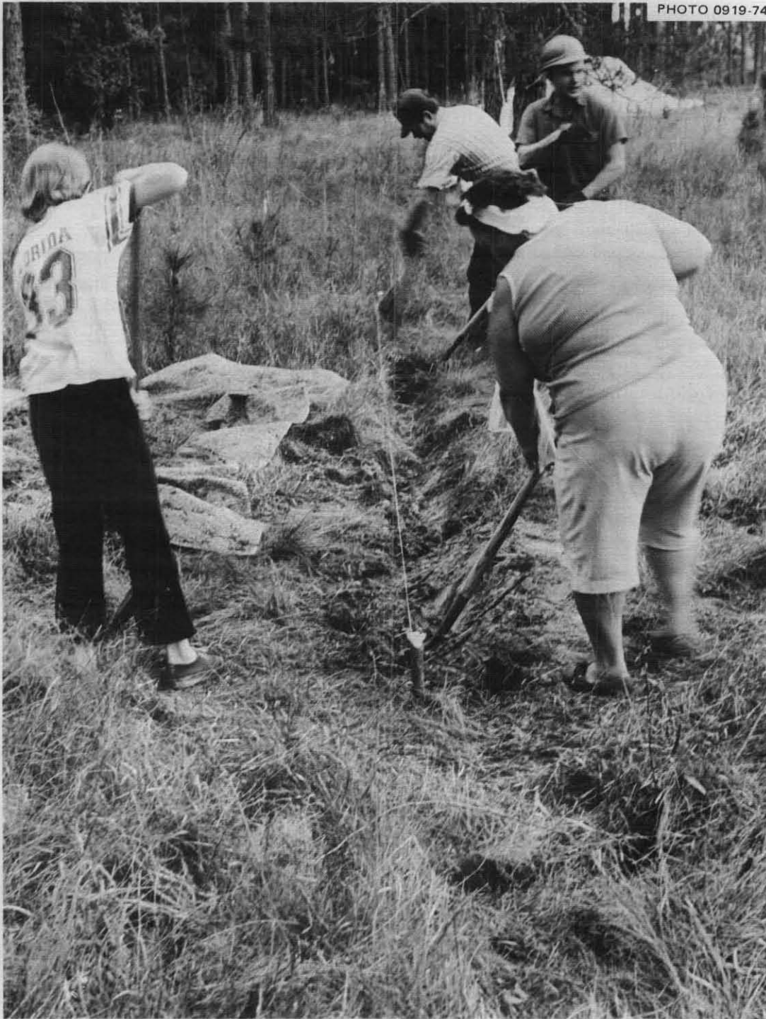
Fig. 5.42. Starting to build a 21-person above-ground A-Frame Pole Shelter. Five families, having 22 persons in all (including two babies and three adults unable to do heavy work) built this shelter with a main room 21 ft by 13 ft wide. The roof poles (not shown) had a minimum small-end diameter of 3\frac{1}{2} in. and sloped approximately 36^\circ . This photograph shows one of the 6-in.-deep, "V"-shaped trenches being dug to secure the lower ends of the 9-ft roof poles, that measured 9 ft on their short sides.
